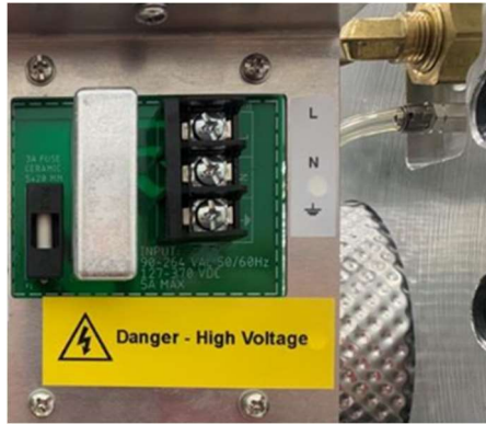
Figure 2-1: Input Power Board
