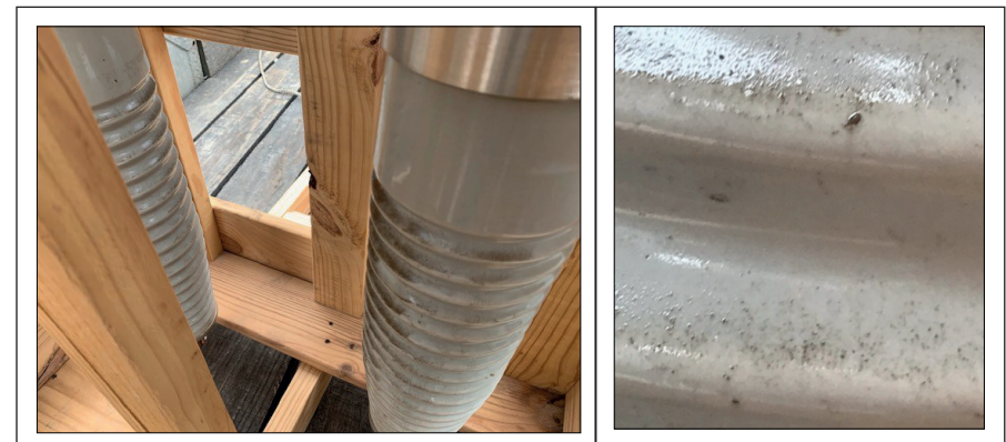
Figure 4: HV bushing removed from the transformer – surface contamination on its lower insulator
