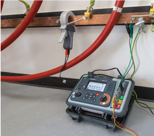
Using ART method with Megger DET2/3 Series to test commercial earth (ground) without disconnecting the system
