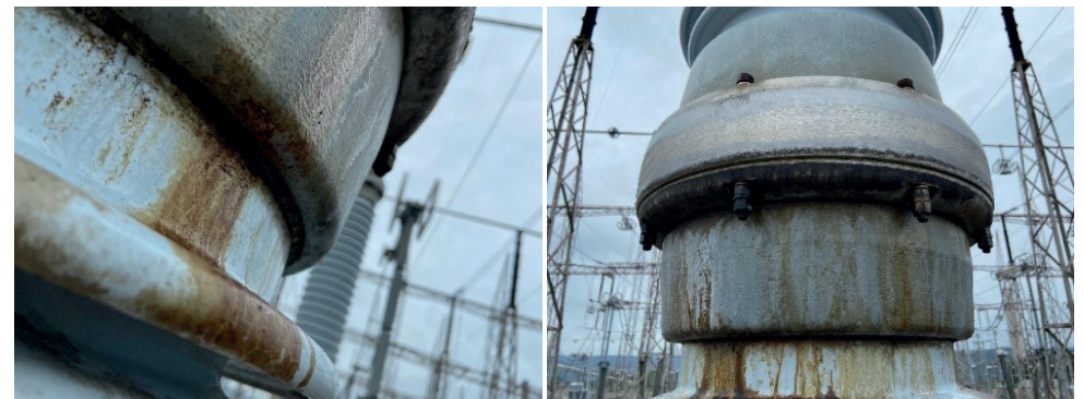
Figure 6: CVT-2 as found during visual inspection
